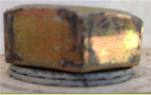
Nordlocks installed back to front.
