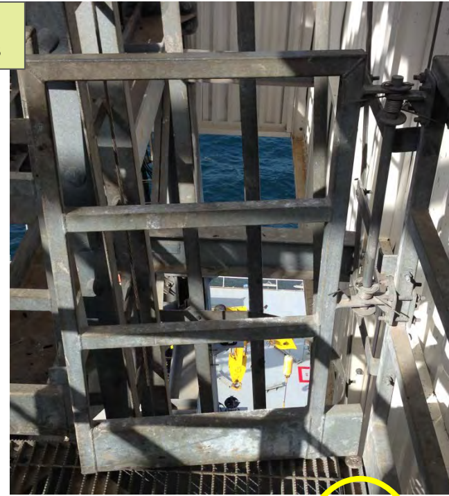
Retention line on housing, not diffuser
