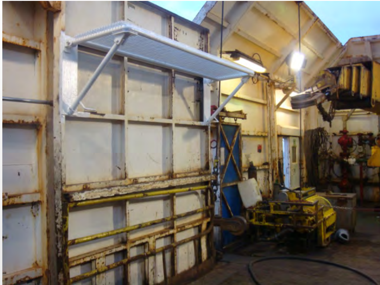
Drill Floor overhead protection
