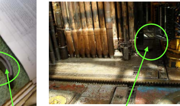
Area where bearing landed.
