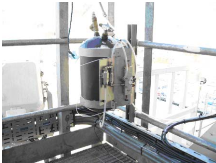
Water flushing tank
