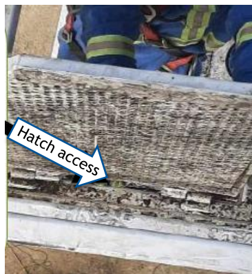
Hatch access area where slip die fell through
